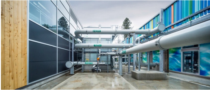
City of Richmond's ADEU energy centre
