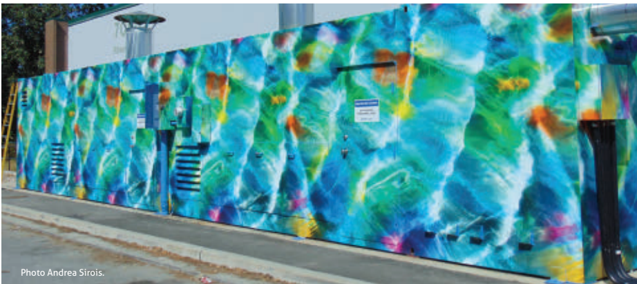
This vinyl mural, Underwater by Andrea Sirois, wraps around the 53-ft shipping container that houses one of the Oval Village system interim plants.
